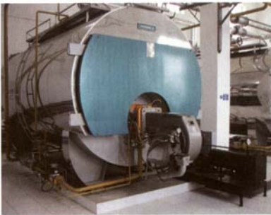
Figure 4b Small boiler.
