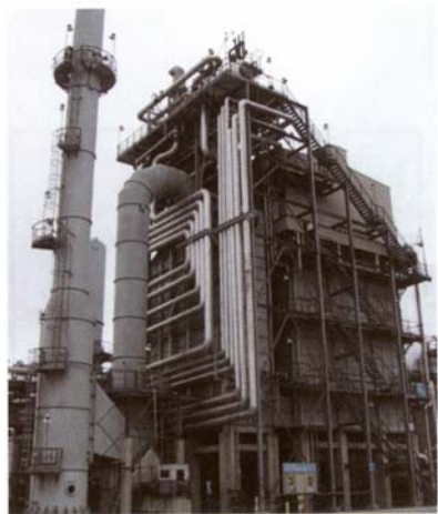
Figure 5b A hydrogen production furnace with burners on top.
