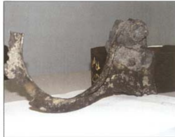
Corroded roof hanger.
